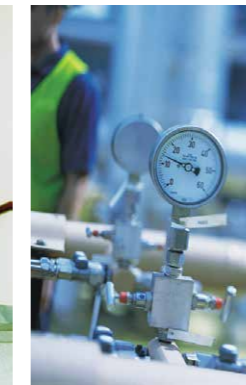
Sprinkler Flow Switch
