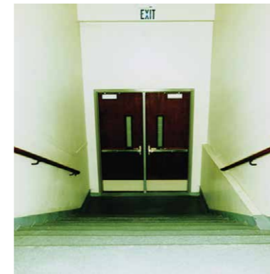
Emergency Exit Monitoring
